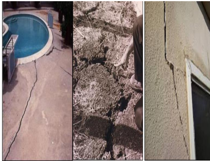
Figure 1. The damage of structures and cracks in expansive soil [4]
