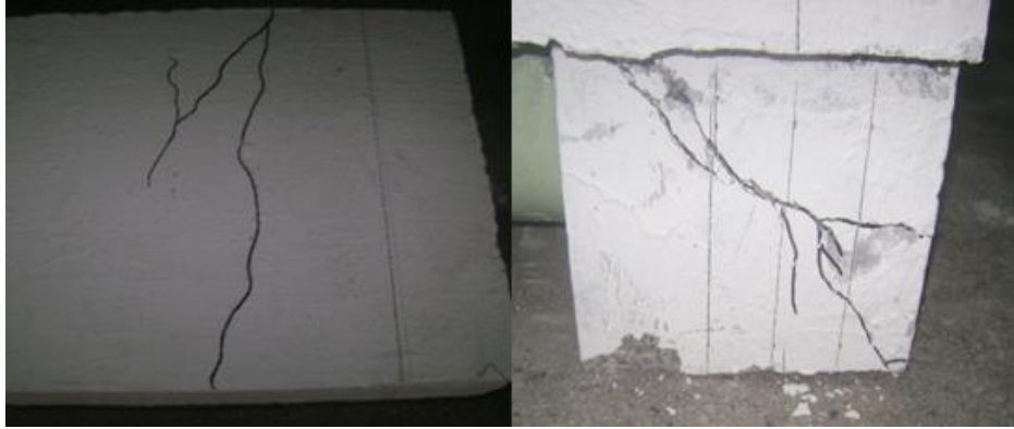
Figure (13): Shear cracks at support in beam CB7.
